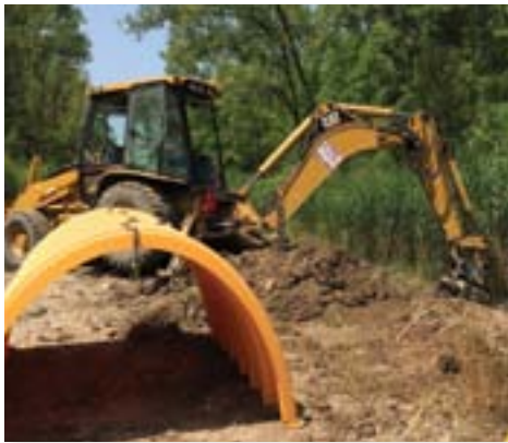
In most cases, access and work by heavy equipment must be sequenced and completed before the final trail prism can be shaped.
