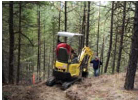
A 37" wide mini-excavator constructs a single track trail and it looks wide and rough.
