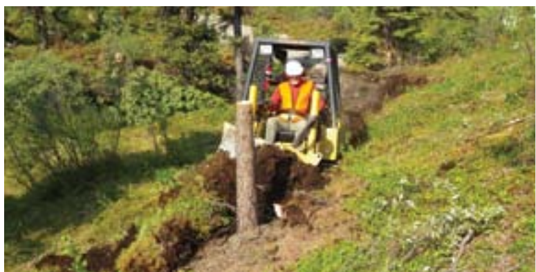
The dozer is removing the organic layer of vegetation and grubbing stumps. Note the high-cut stump for increased visibility and leverage.
