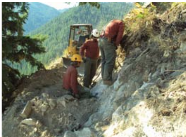
The deeper the cut, the higher the likelihood of encountering solid rock. Having air tool capabilities makes this less of an obstacle.
