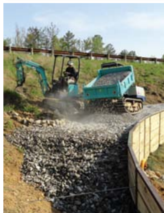
Failure to adhere to specifications on a complex trail like this can result in structure failure, resource impacts, and the loss of a considerable investment.
