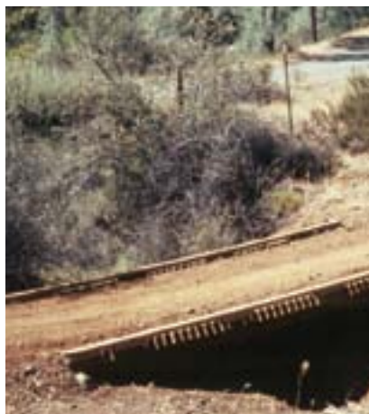
This bridge is in the bottom of a grade sag so water and sediment collect and drain in the middle of the bridge. When this creek is flowing, sediment will be delivered directly into the water. If this was a perennial, fish-bearing stream, this bridge site would not be acceptable.
