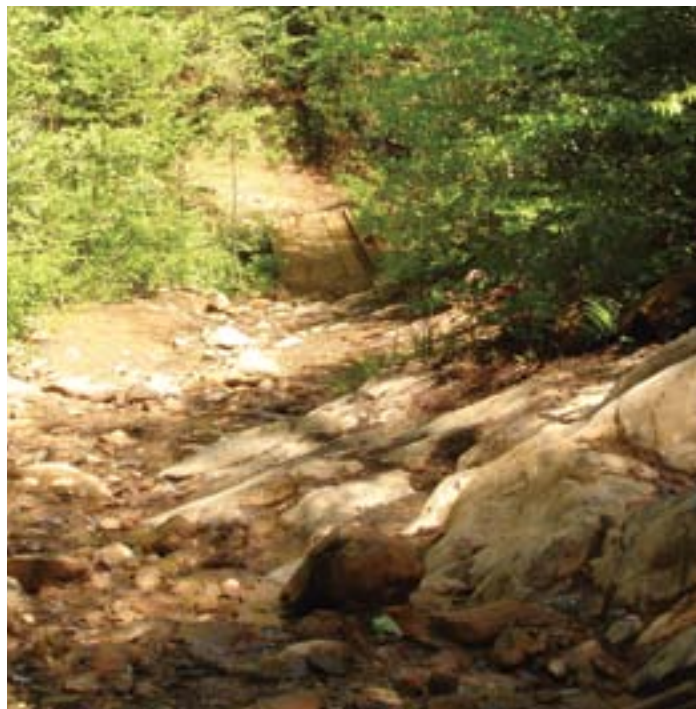
This is a common, but poor bridge approach. This long grade has no drain. All of the water and sediment will be deposited directly into the creek. Vehicles trying to brake going down or accelerate going up will churn up more soil that will also end up in the creek. Old roads are often used for bridge access because they are existing and provide a means to get equipment and materials into the bridge site. This is okay, but using the road as a trail afterward isn't. A properly designed trail should be located and constructed and the old road closed.
