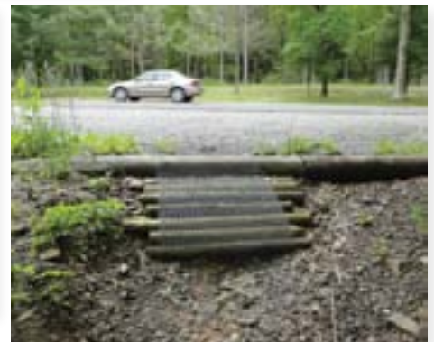
Manage parking lot drainage through design. The low point of this lot is at the trail access point so all of the water flows down the trail. Attempts to harden it will be futile and the best option is to relocate the trail access point.
