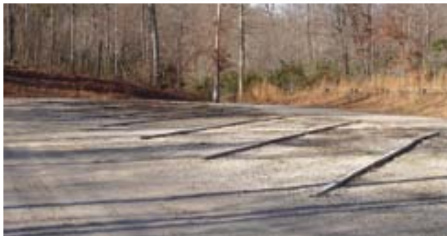
These treated timber parking delineators are expensive, inhibit parking lot maintenance, and don't work well to organize the parking. People will be driving over them and tripping over them. A Park in Center sign would help. The angle of the parking should be determined by the angle to the parking lot entrance. If it isn't, one row of timbers would be sufficient to guide the first vehicle.
