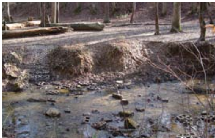
Pavers must be properly bedded and anchored or they will fail. Note the creekbed littered with pavers. There should be one approach to the creek, not three. A ford constructed of concrete planks cabled together would have worked better.
