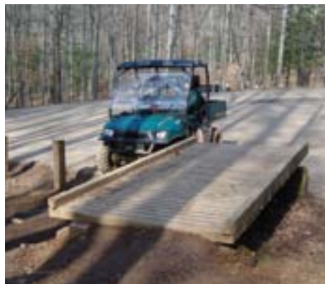
This is a nice ramp, but weather and tire action are eroding the approaches. They need to be hardened to keep it functional.
