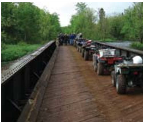
The opportunity to use this old railroad bridge as an OHV trail enhances the rider experience and saves project dollars. This could be a good place for some interpretation as well.
