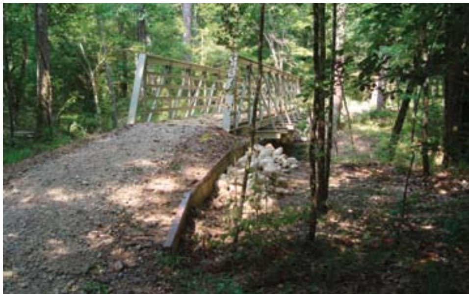
This is an excellent bridge approach. Raising the trail grade to the bridge forces water off the trail and helps prevent dirt and rock deposits on the bridge deck. Water drained off the trail has plenty of natural vegetation to flow through before entering the stream. This will slow the velocity and filter out sediment.
