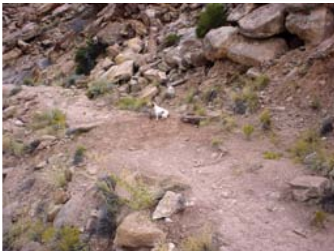
A newly constructed rock waterbar with a smooth approach. (Note: these will work if the rocks are large and well-embedded to resist the tire impact forces.)
