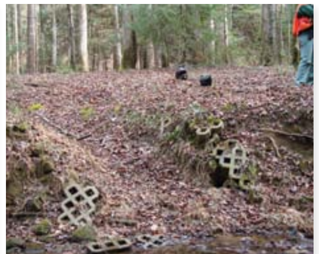
Poor paver installation in this stream crossing resulted in resource impacts. Cobble stone would have been a better choice.
