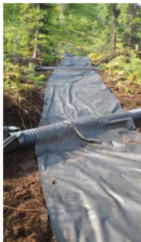
Geotextile is being put down to provide separation and reinforcement on this Alaska trail.
