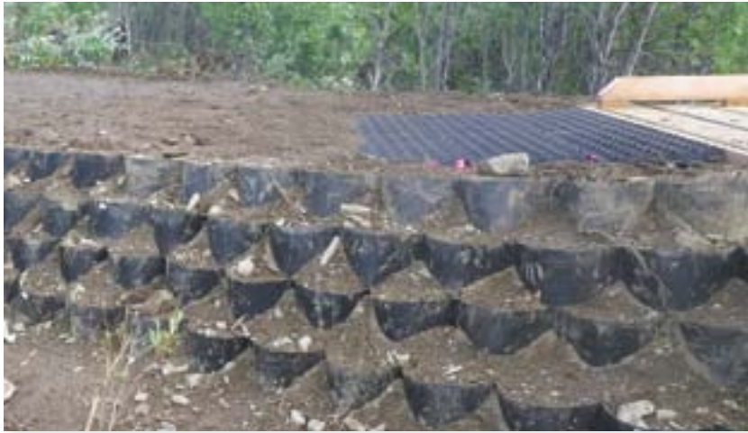
The fill for this bridge approach and bridge abutments has been constructed in layers of geocell with a good soil and rock mix. Note the grass paver panels to insure a smooth transition onto the bridge deck.
