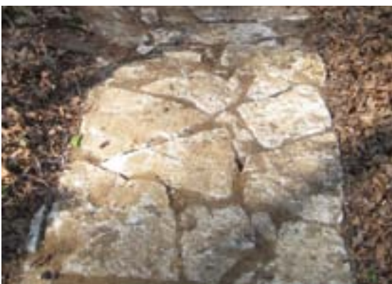
This hardening installation is composed of chunks of sidewalk that was headed for the landfill. Being heavy and angular, the pieces should key together very well. Notice that they have been embedded so that the edges are contained by the natural soil.
