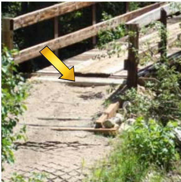
This geocell bridge approach is in the process of disintegrating. Bridges and other structures can be very slippery. Having an approach on a curve is not desirable since the vehicles are still on the curve once they hit the bridge deck which increases the risk of losing control and sliding into the railing. The curve also creates more lateral tire forces which act to increase displacement on the geocell and deck approach. Note the lip on the bridge abutment (arrow). This will bounce a motorcycle tire off the ground and increase the risk of sliding on the bridge deck.
