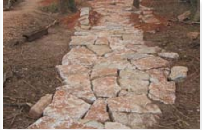
These rock slabs are well-placed and keyed together, but they lack confinement. Rotational and centrifugal forces will gradually displace them.
