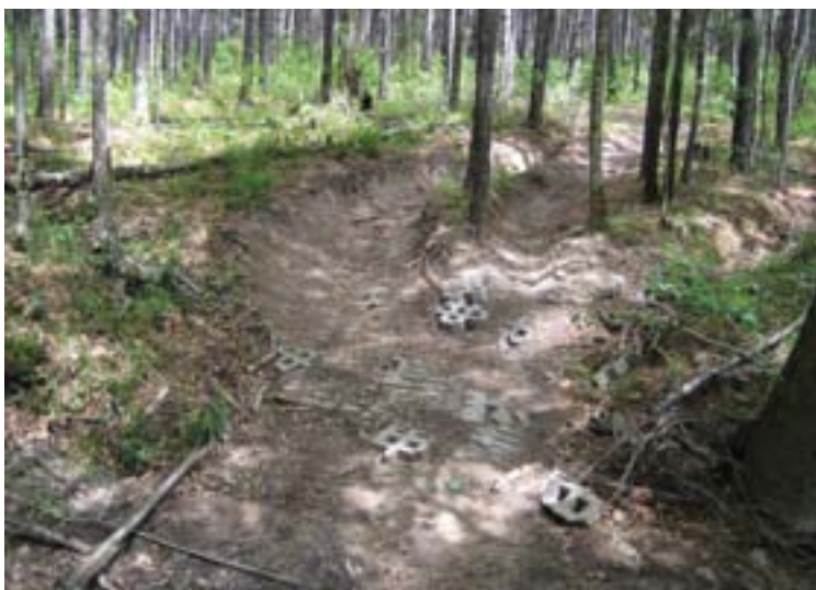
The results of a poor installation: broken pavers, two eroded trenches instead of one, risk, resource impacts, and a mess.
