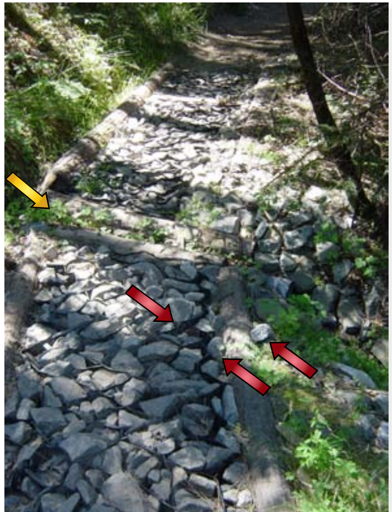
This is an excellent example of a trail hardening installation that will likely fail. On the plus side, the material is framed into sections which help prevent movement. The gap between these two sections (yellow arrow) serves as a log culvert. On the minus side, this cobble surface is rough to ride on and the rotation action of the tires will displace the rocks out of the Geocell (red arrow) and the exposed cells will start to break down. The life and functionality of this structure could have been extended if it had been covered with a layer of well-graded aggregate.
