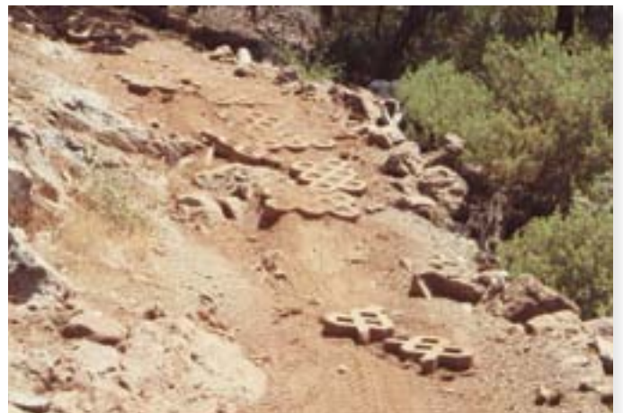
Pavers poorly bedded and placed on an uneven surface of rocks will move and fail.
