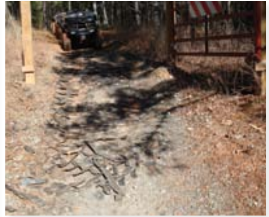
The fill layer over this installation was not maintained. Direct tire impact displaced the material in the cells and destroyed the integrity of the structure.
