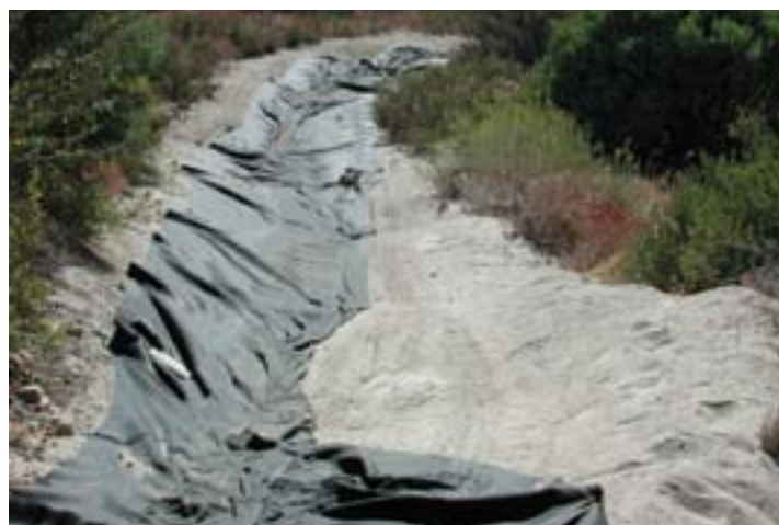
Tires and geotextile do not mix.
