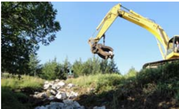
Need more reach? Not a problem as this excavator places a blanket of energy dissipaters in this drainage.
