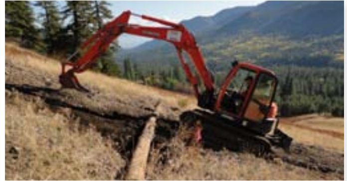
This excavator is rehabbing old hillclimb trails. It is scarifying the trail, installing waterbars in a herringbone pattern, and strategically placing logs that divert water and deter riders.
