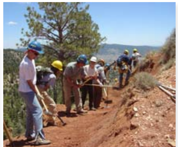
Camaraderie is important with any crew, but this group is working too closely together for safety. There should be a minimum of 6' between workers. It is a good example of the use of hardhats and the number of tools that are needed for a work crew.
