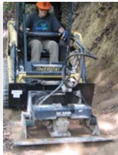
These handy vibratory plates will not exert the same compactive effort as a smooth drum roller, but they do a good job smoothing and compacting the surface of the tread. One advantage of compaction attachments is that they can be raised by the equipment to avoid root or rock sections.
