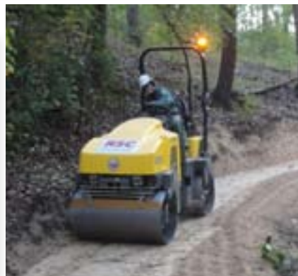
Moist soil will compact better than dry soil, so try to time compaction operations during periods of favorable moisture content.
