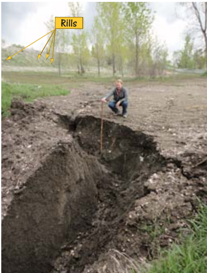
This is a view of the bottom of a large tread watershed. The soils on this site are very poor. When the spring storms started, so did the erosion. Though grassed in, look at the rills on the slope that are feeding water to this drainage point.
