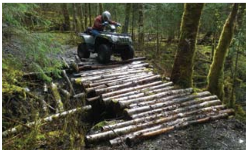
In the backcountry, corduroy is sometimes used as a bridge. This is not a recommended practice and should be considered a temporary bandage due to its structural instability. Grade should be avoided with corduroy, especially in wet climates. The slippery, uneven logs on this installation make it a liability.
