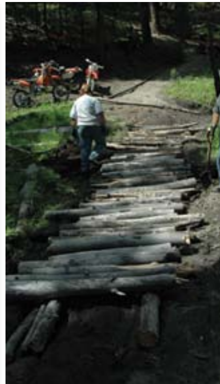
Corduroy anchored onto stringers will last longer and create a more stable tread. This is an example of a poor quality installation. The stringers already show signs of rot and the corduroy logs should have been cut into even lengths.
