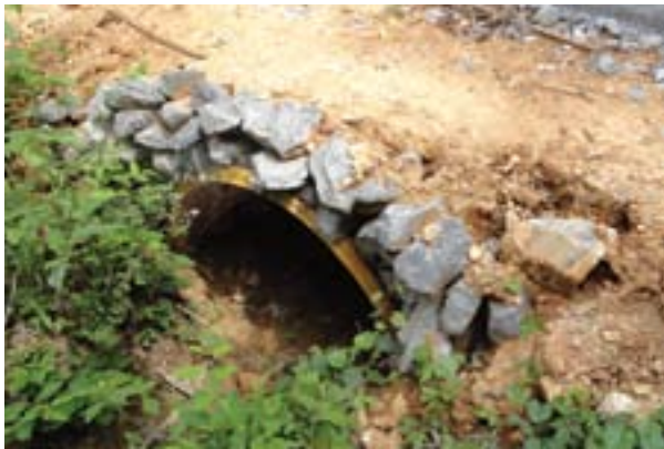
Culvert headwalls are always a nice touch. This rock headwall supports the trail fill.
