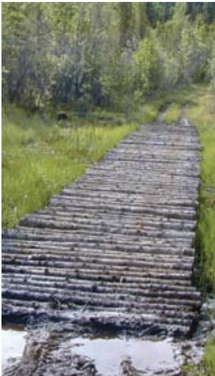
This is nicely constructed with poles of the same length and diameter. Unfortunately, it isn't long enough. This is a common and costly problem with many tread structures.
