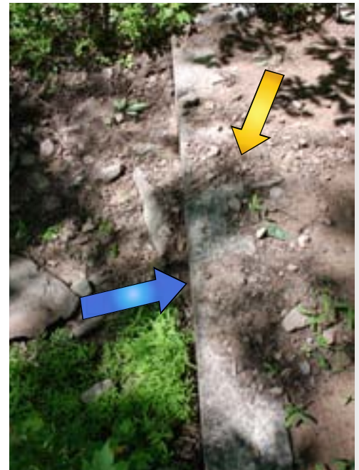
This treated timber waterbar provides a formidable obstacle from below (blue arrow) and being full of sediment, it provides ineffective drainage (yellow arrow). The issue: the tread watershed is too large. Poor soils cannot sustain this grade that is too steep for too long. The solution: relocation.
