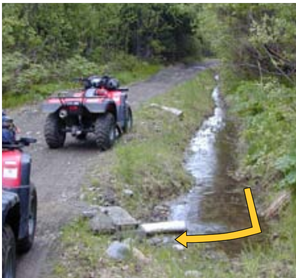
Note how water is running past this culvert rather than flowing into it. This installation would be more effective if there was a rock catchbasin to help turn the water into the culvert.
