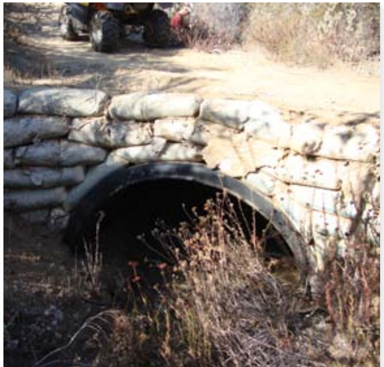
As the wrappers fall off, a pre-mix headwall can look a little shoddy, but that is temporary. To avoid that, the wrappers can be torched off after the concrete has set.
