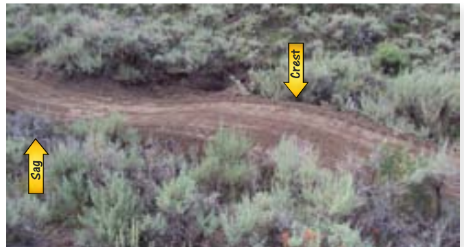
This is a nicely constructed rolling dip. Notice the distance from the sag to the crest and notice how the grade smoothly rolls into and out of the dip.
