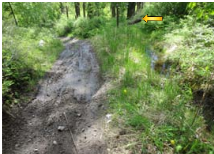
Water will always take the path of least resistance. A mudhole developed by water from this spring saturating the soil below it. A ditch was cut towards the log (arrow) to drain the spring water away from the trail. There was a layer of solid rock that prevented the ditch from being cut lower than the trail tread, so even though some water flows down the ditch, gravity will still pull water down the impermeable rock layer and into the trail. An alternative is to blast the ditch lower or install a French drain in the trail.
