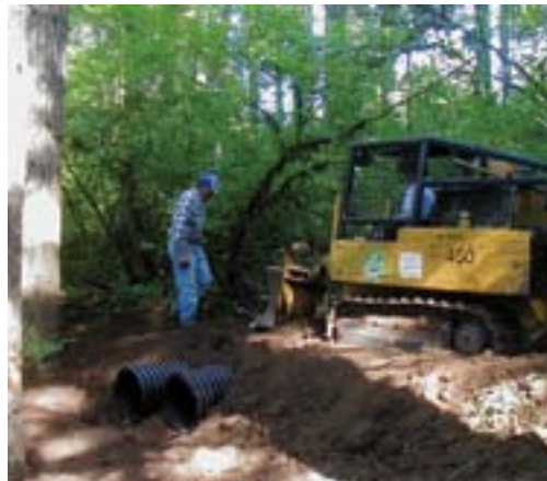
It is dry now, but this runs a lot of water in the winter. Two plastic pipes in this shallow drainage keep the trail fill low and provide a safety net to handle unusually heavy flows. Two pipes have to be carefully bedded to prevent water from running between them.
