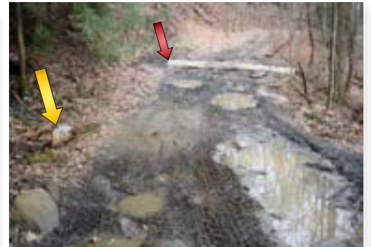
The first culvert (yellow arrow) was properly installed in the drainage. The second culvert was added later possibly to drain a spring but was not installed properly due to rocky ground. Manage your risk. The second culvert does nothing but create a safety hazard and an opportunity to ruin what was a good section of culvert. A side ditch draining into the first culvert may have been a better solution here.
