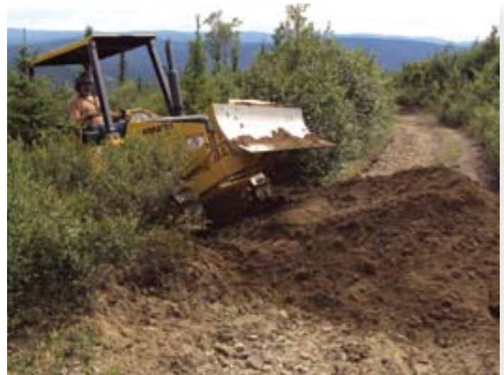
The best way to start building a rolling dip is to borrow as much material for the crest as possible by using lead-off ditch or drainage sump excavation. Excavating the sag to build up the crest increases the grade going into the dip, reduces the flow of the dip, and can make it more difficult to drain water out of the dip.
